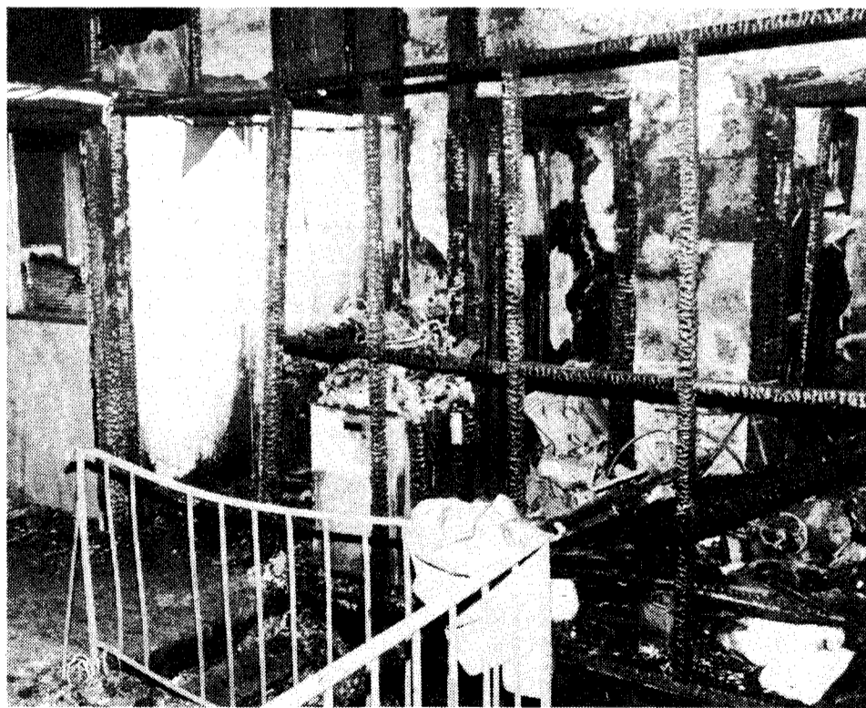
SWP headquarters after fire.
