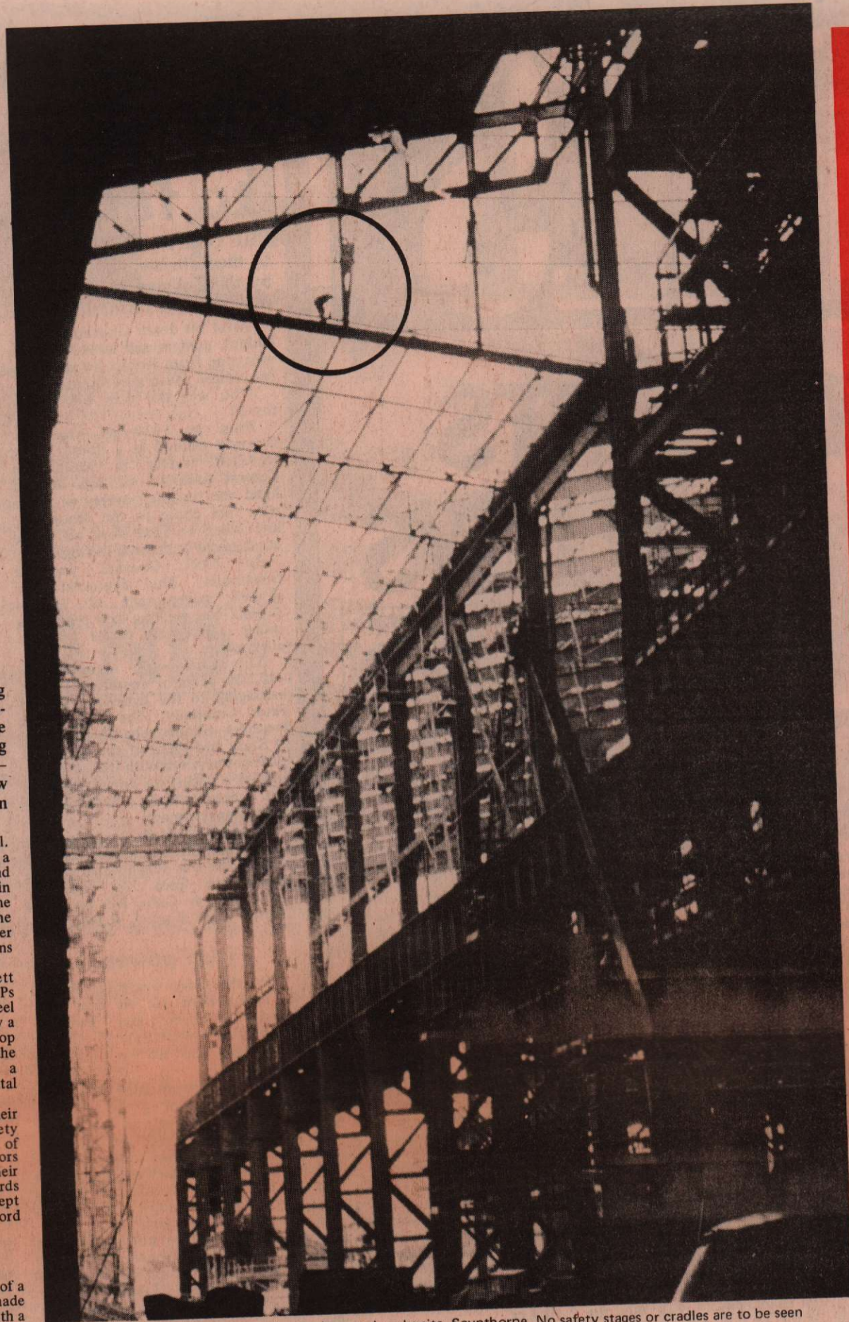
Painters at work on roof beams at the Anchor steelworks site, Scunthorpe. No safety stages or cradles are to be seen
