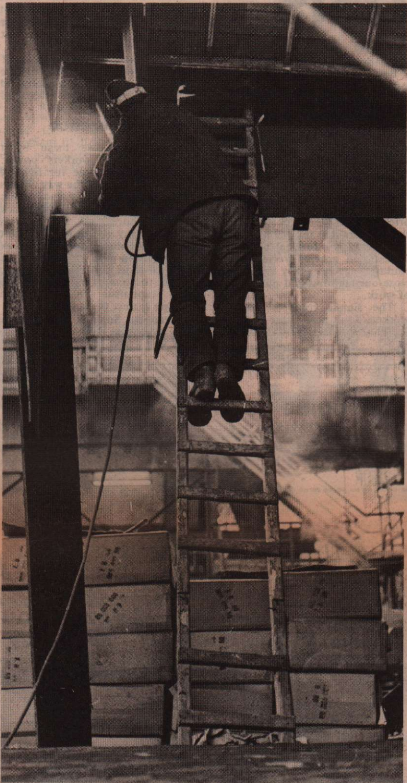
The ladder is unsecured and has a rung missing. One false step and this welder could fall on blowtorch. PICTURE: Christopher Davies (Report)
