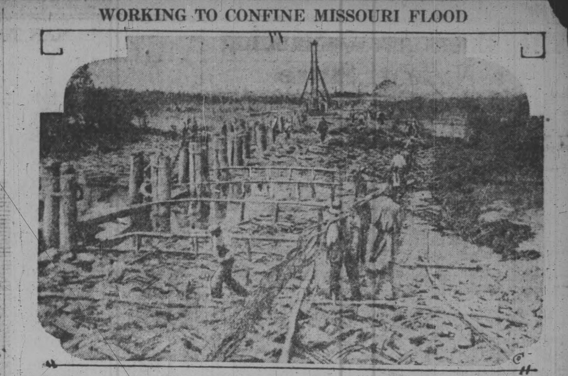
Workmen are driving piles and putting down willow mats to try and confine the Missouri River to its old banks. Picture is taken at Sny Bend, near Lexington, Mo. Pretty late to help the flooded regions.
