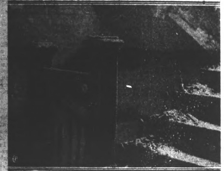
Here is a photo in the interior of the Graystone Apartments, Indianapolis, Ind., where an early morning fire caused the death of eight persons and the serious injury of 14. It shows the burned stairway. The only fire escape in the building adjoined the only elevator shaft. This was in defiance of safety laws, but some influence passed this and other buildings in Indianapolis. When fire broke out, both elevator and fire escape burned at once.
