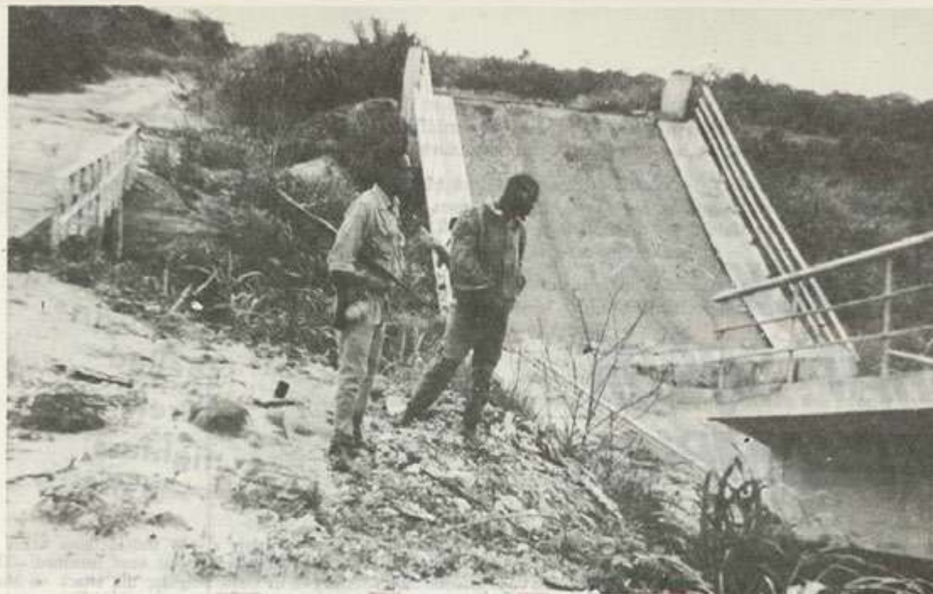
Another bridge blown up. This one was in Niassa Province
