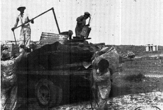
A lorry carrying Korsten shacks being offloaded at the Site and Service area.
