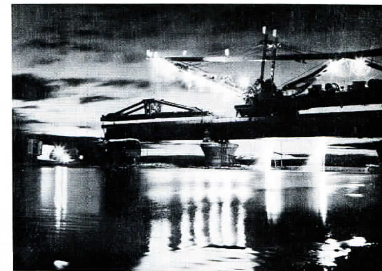
Building a bridge over the Buh River on the Qinghai-Tibet railway line.
