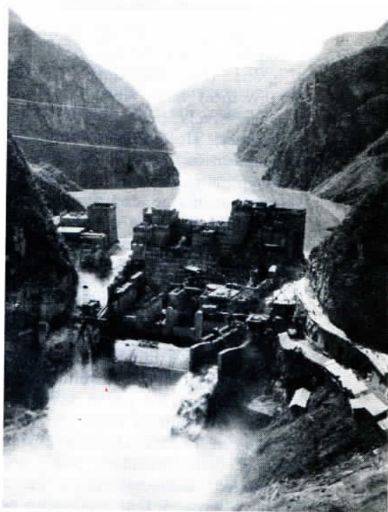
Construction of the Wujiangdu hydroelectric power station in Guizhou Province (with a capacity of 630,000 kilowatts) is under way.
