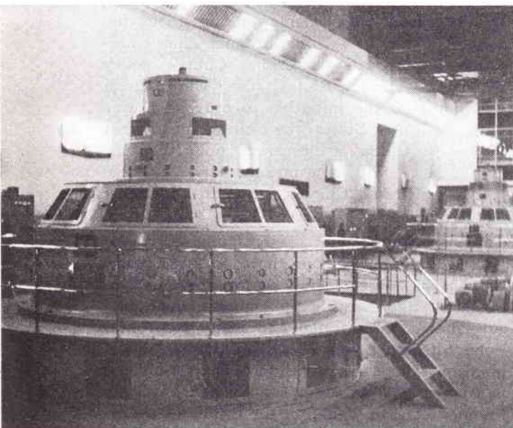
The No. 2 generating unit of the Wujiangdu Hydro-power Station has gone into operation.
