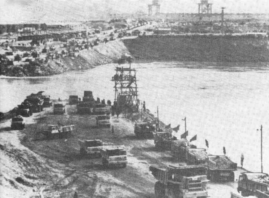
A cofferdam being completed across the Changjiang River at Gezhouba where a water-conservancy key project is under construction.
