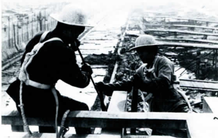
The first-stage of construction on the Huaian double-course ship lock, part of the project to divert water from south to north.
