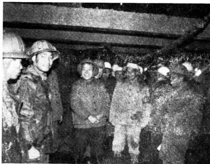
Mayor Li (centre) joins PLA construction crews in the tunnel of the Luanhe River project.
