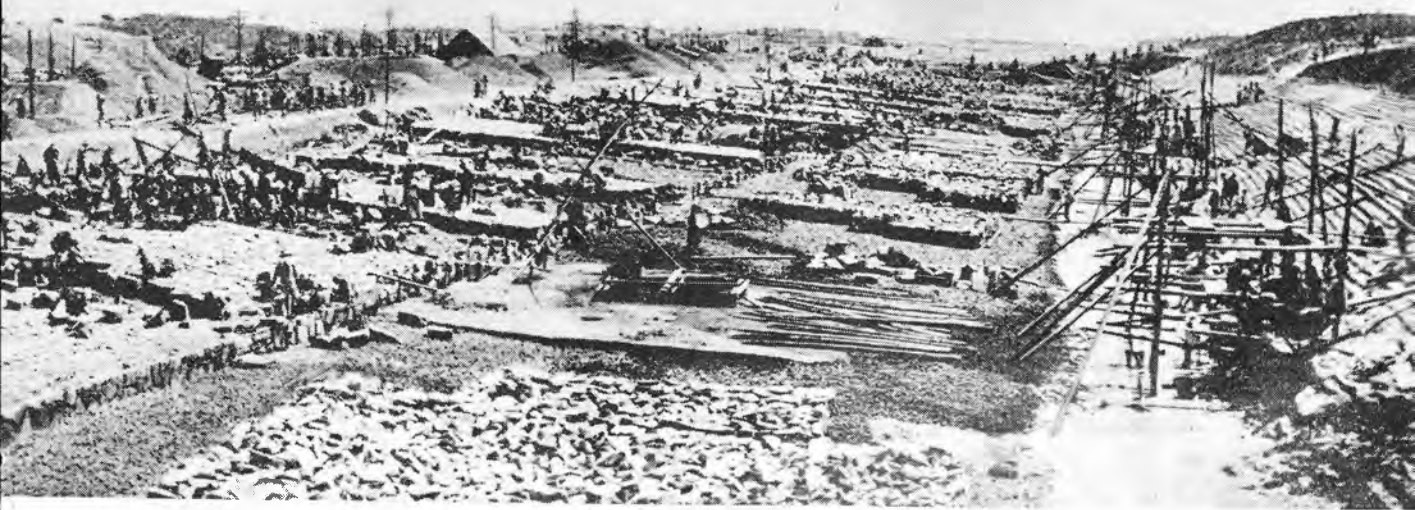
Work on the Jenhochi Dam on the Huai River in Anhwei Province, one of the biggest projects
