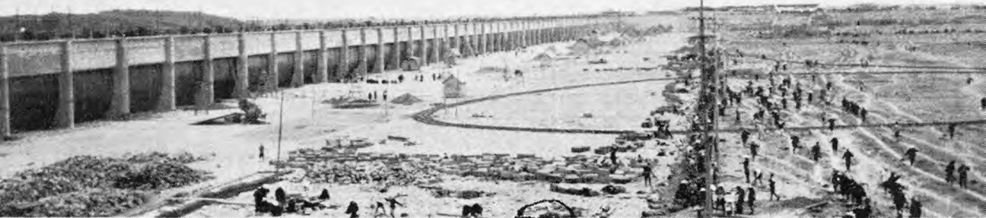
Workers laying stonework on the river bed near the 697-metre-long San River Regulating Dam
