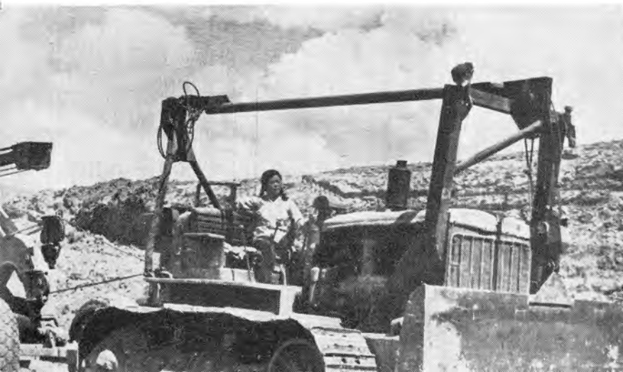
Signs of the times in the Northwest. Hu Yu-mei, a woman bulldozer operator on the Tien-shui-Lanchow Railway construction site
