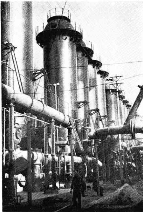
Reconditioned Cowper stove for heating the air blast at the Maanshan Iron Smelting Plant (Anhui Province). Six blast furnaces have been recommissioned here after being out of use for over eight years
