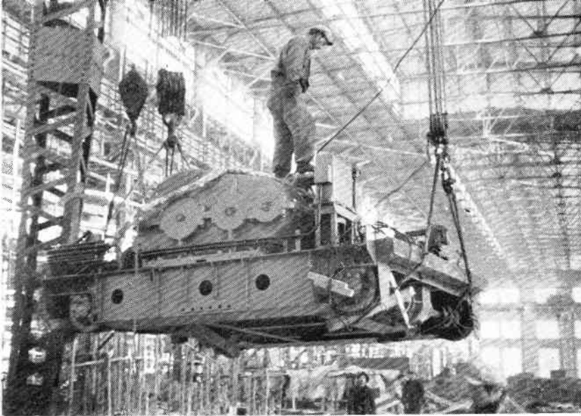
Installing a giant machine in the Harbin Electrical Machinery Plant, which will soon go into production
