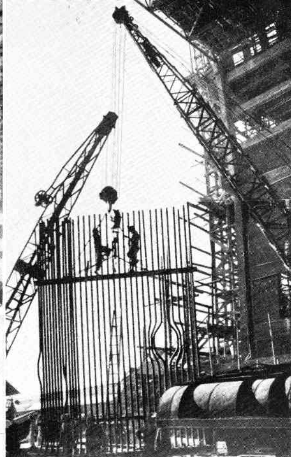
Assembling water-cooling pipes in the boiler room of Chungking's No. 507 automatic power plant, the first of its kind in Southwest China. It was commissioned in April this year
